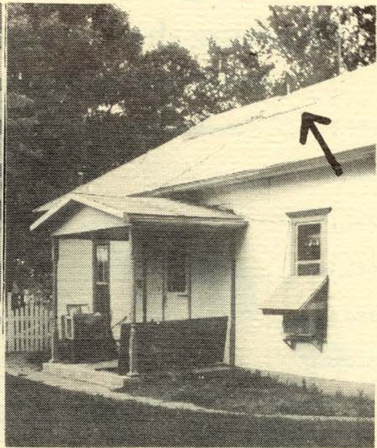
Note solar hot water panels on roof.
