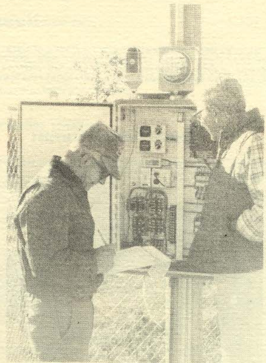
Harlan Johnson, Water-Waste Water Coordinator and Bob Sanders, Mayor of Ohioa, inspect part of the waste water facility installed just outside the rural community. Pictured is the two cell lagoon and the control and alarm system for lift station.
